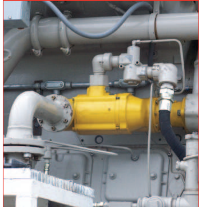
The ST1099CP03R25 is piped for use on a Waukesha 7044 gas compression package.
